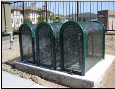
EXPANDED METAL ENCLOSURE (SECURITY)
