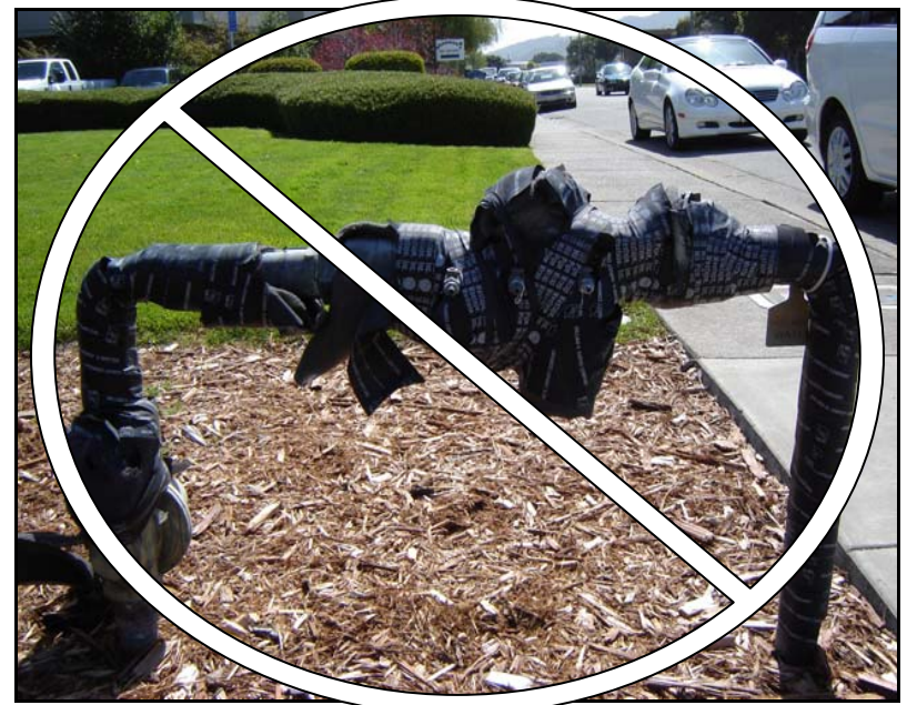
UNAPPROVED METHOD OF PROTECTION
