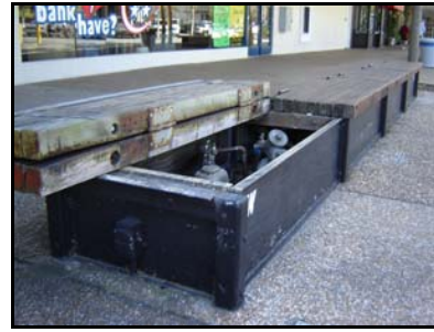
CUSTOM ENCLOSURE (SECURITY)
