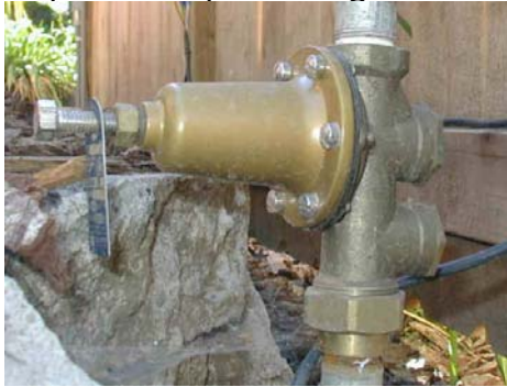
Mainline pressure regulator
