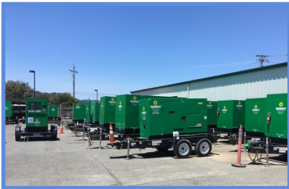
Image 5-2: Rental Generators Staged in Anticipation of a Public Safety Power Shutoff
