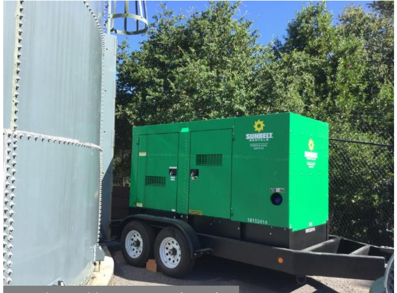
Rental Portable Generator (2020)
