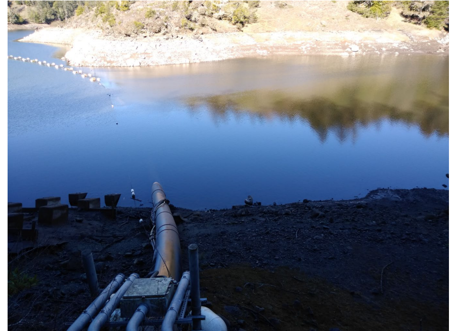
Alpine Lake Pump discharge
