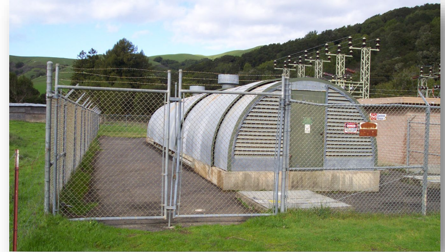
Tocaloma Pump Station
