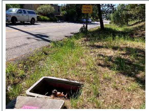
South Alignment's connection to the existing recycled water system on the north side of Merrydale Road south of North San Pedro Road looking north.
