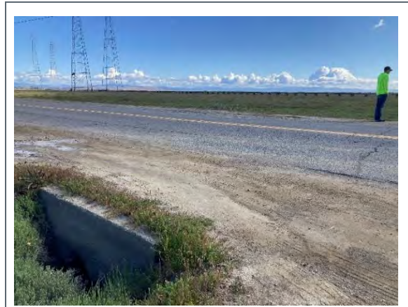
Culvert crossing is very shallow under North San Pedro Road.
