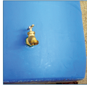
Figure 17. Hose bib facing down.
