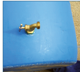
Figure 18. Hose bib facing to the side.
