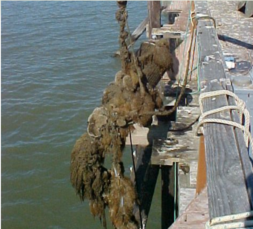
Intake after three months with no cleaning from April to June 2006
