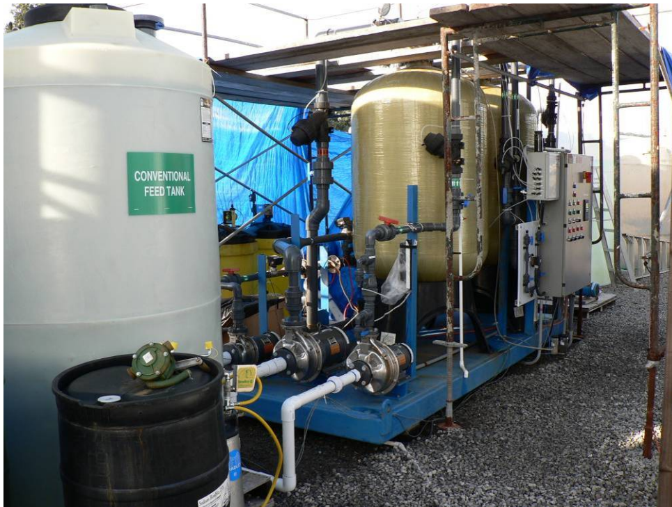
Conventional pretreatment system filters
