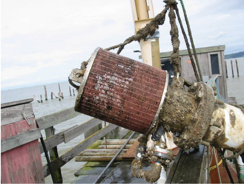
Intake screen after manual cleaning 3 April 2006
