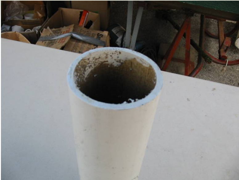
Thin bio-film on intake pipe after three months operation
